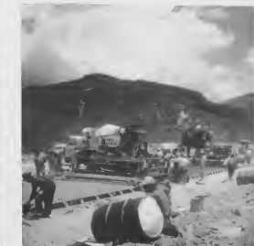
Reinforced cement with an asphalt cap makes the surface of the new highway all purpose. The two double lane sections are separated. Along both sides of the highway are cement shoulders.
